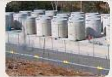
Spent fuel storage
